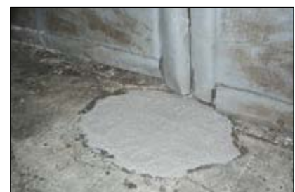
Figure on top: Deutsche See GmbH & Co. KG, Bremerhaven: Repair of floor areas in cold store house with SILIKAL® R 17 mortar with no disruption to operation (-25 °C)
